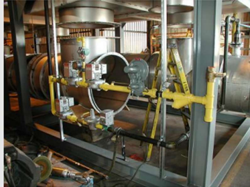
Additional Fuel Train Piping
